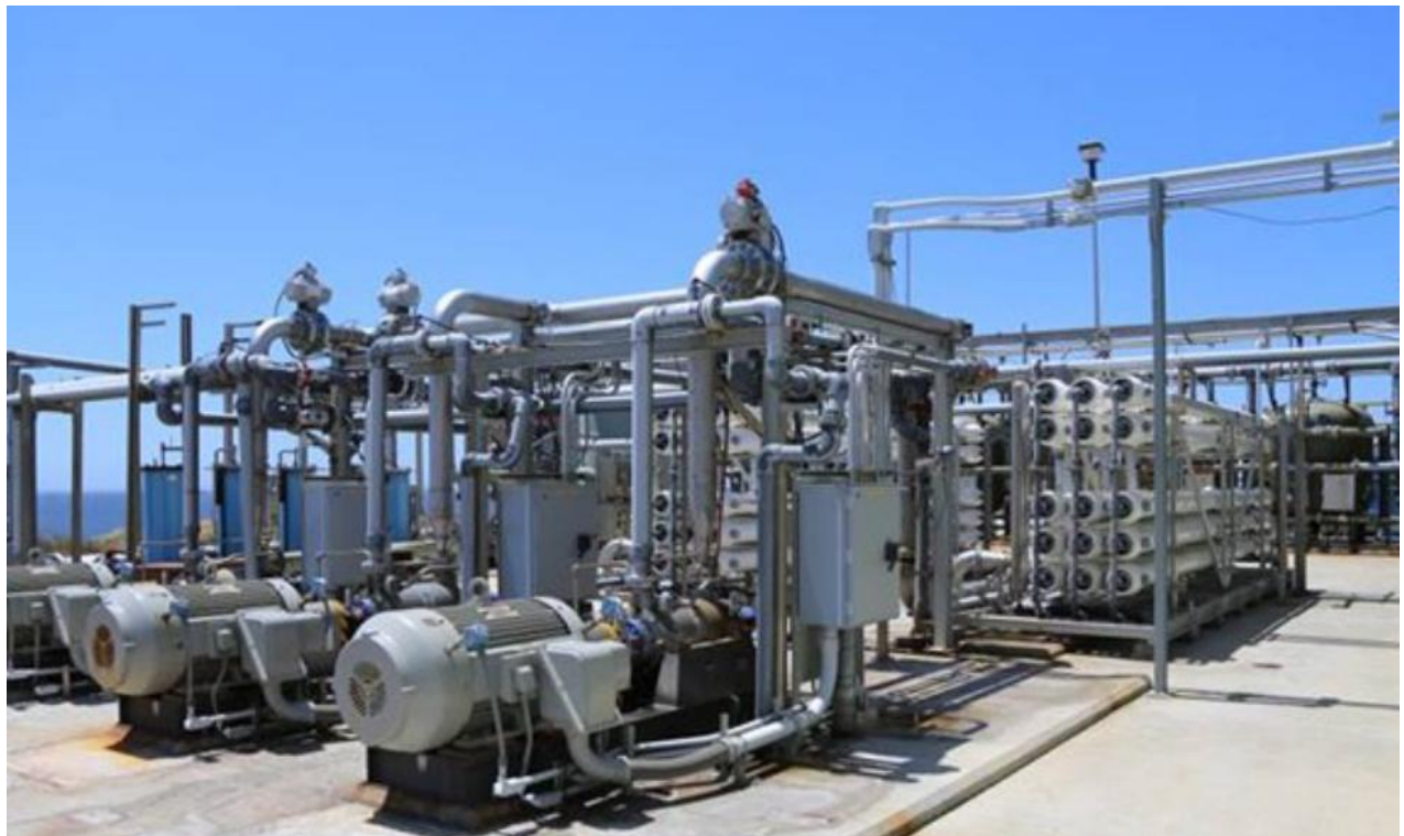
Existing desal infrastructure currently in place and functioning at Diablo.
